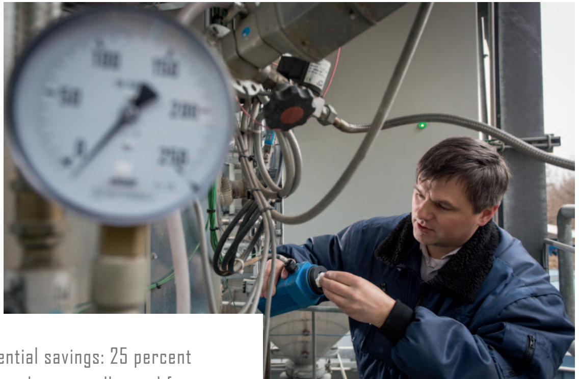
Bernhard Kiep at work on the experimental plant in Gerstungen.
